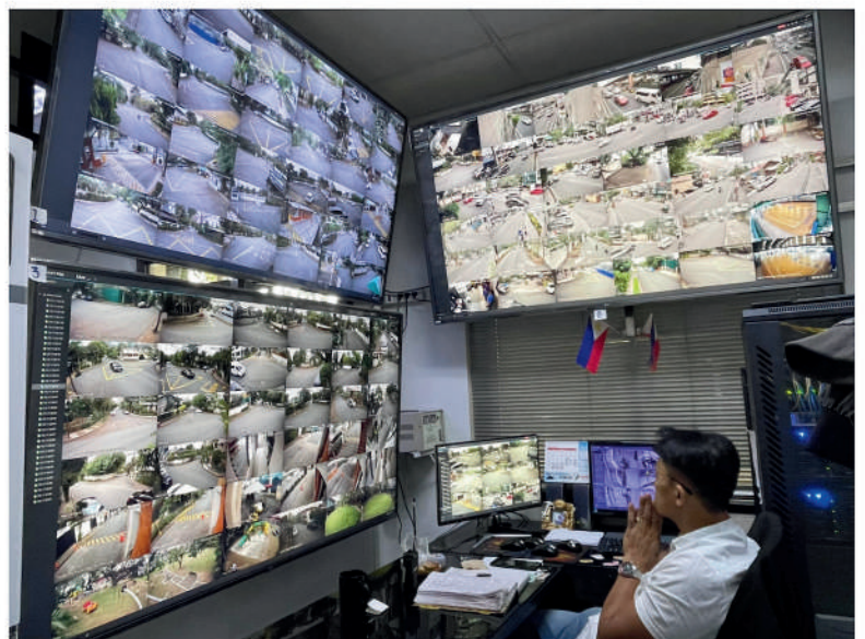
BEL-AIR VILLAGE CCTV ROOM
