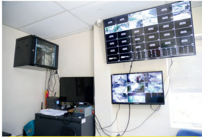
SALCEDO VILLAGE CCTV ROOM
