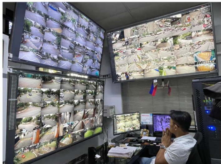
BEL-AIR VILLAGE CCTV ROOM
