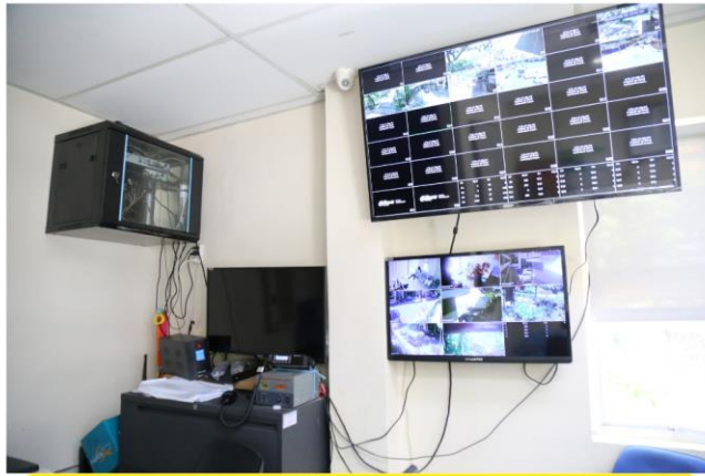
SALCEDO VILLAGE CCTV ROOM
